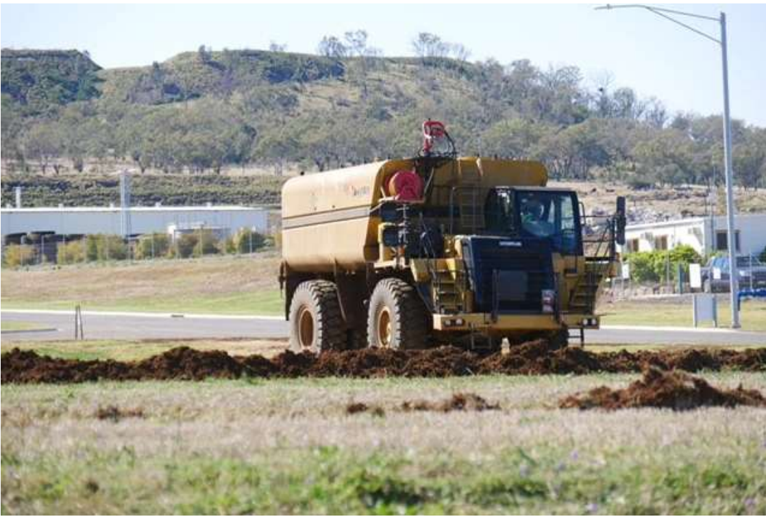
Work has started at the Wellcamp Business Park site. (ABC News: David Chen)
